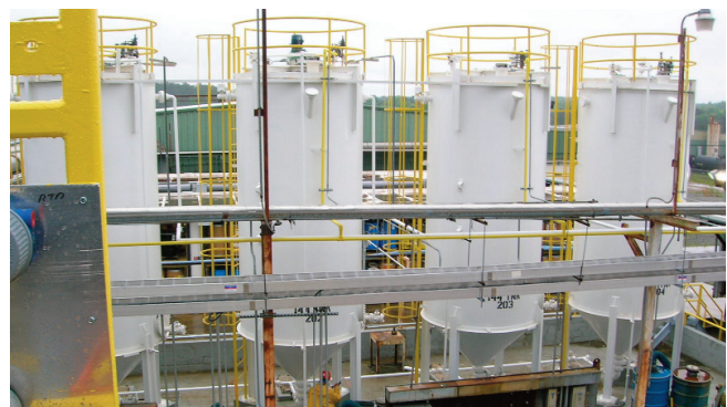
Solvent Recycling Tank Farm
