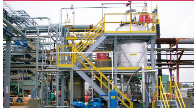
Vacuum Distillation Unit
